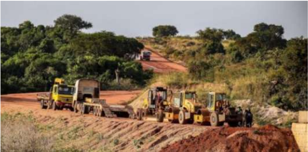
Figure 52. Bulldozers and compactors line up on the road construction project stretching from Tangi gate to the Nile River bridge crossing. This road extends through the heart of the park and will facilitate large tankers in their oil delivery activities. Photograph: Alamy.
